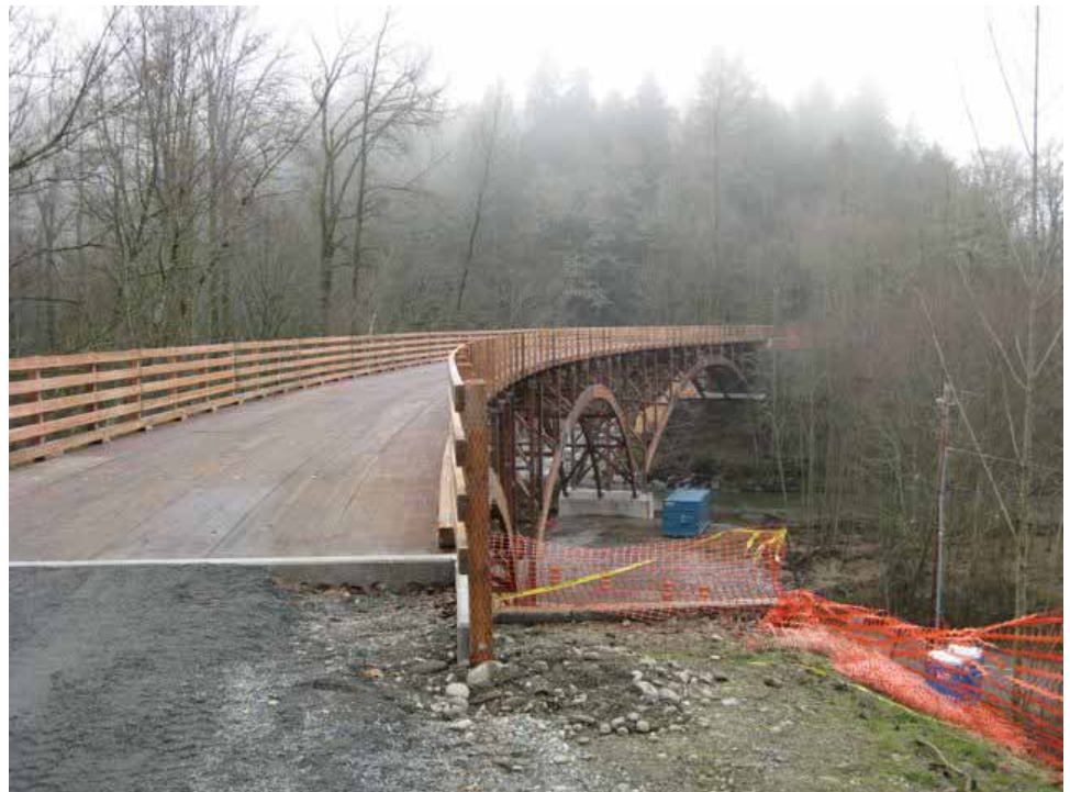
Right: The decking has not been paved yet but can be ridden without any problem"
